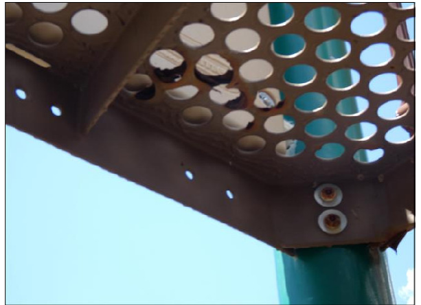
Playground, Note Rust
