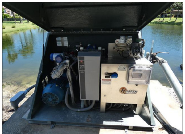
Pump Station 1 Montecito Dr
