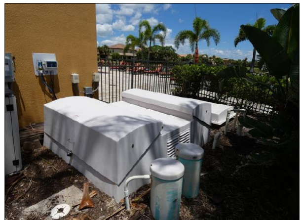
Pool Equipment Housing Boxes
