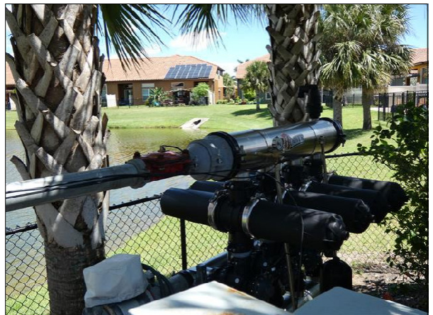
Pump Station 3 Carlsbad Dr
