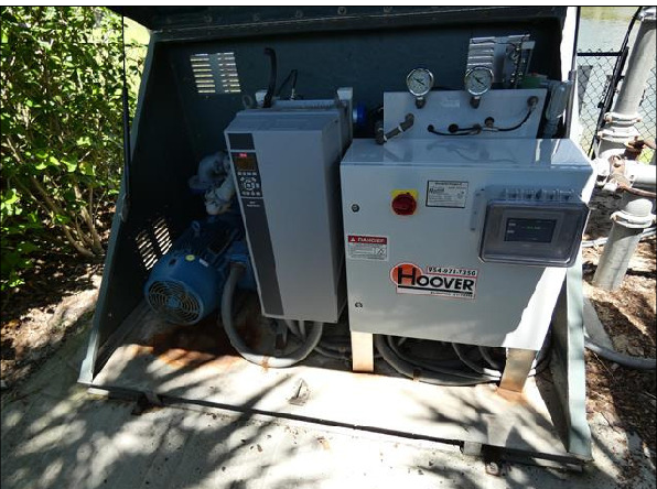
Pump Station 3 Carlsbad Dr
