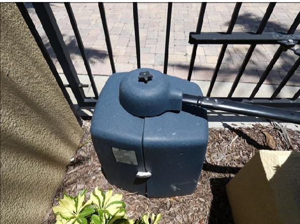
Palisades Dr Gate Operators
